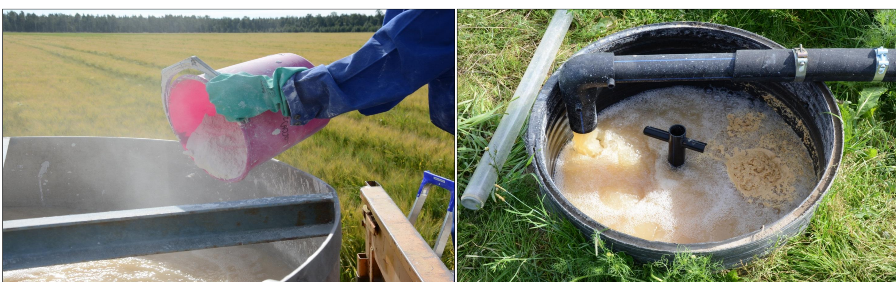
Figure 3. On the left: Preparing of the suspension in a mixing container. On the right: Injection of the suspension via the control well into the drain pipes. Each treatment were performed on two subfields during summer droughts. Treatments in 2012: c. 700 kg \text{CaCO}_3 and c. 150 kg of \text{Ca(OH)}_2 mixed with 100 m 3 water and in 2013: c. 370 kg of \text{CaCO}_3 and c. 360 of \text{Ca(OH)}_2 mixed with 120 m 3 water.
